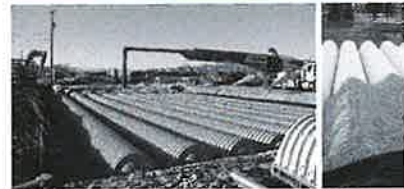
Initial embedment shall be spotted along the centerline of the chamber evenly anchoring the lower portion of the chamber. This is best accomplished with a stone conveyor or excavator reaching along the row.
