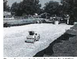
Place clean, crushed, angular stone foundation 6" (150 mm) min. Compact to achieve a flat surface.
