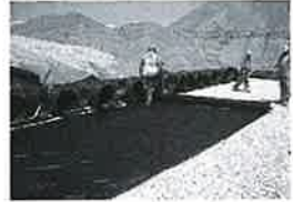
Install manifolds and lay out woven scour geo textile at inlet rows (min. 12.5 ft (3.8 m)) at each inlet end cap. Place a continuous piece (no seams, double layer) along entire length of Isolator® Rows).
