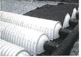
Align the first chamber and end cap of each row with inlet pipes. Contractor may choose to postpone stone placement around end chambers and leave ends of rows open for easy inspection of chambers during the backfill process.
