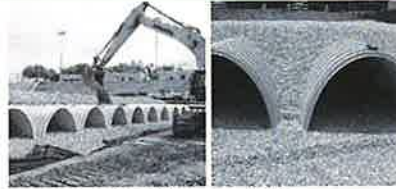
No equipment shall be operated on the bed at this stage of the installation. Excavators must be located off the bed. Dump trucks shall not dump stone directly on to the bed. Dozers or loaders are not allowed on the bed at this time.
